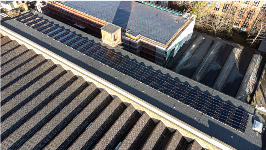
Figure 19: 70 kWp photovoltaic plant installed on Hall 10 of the Leipziger Baumwollspinnerei, © Knut Maurive, Cenero Energy GmbH)
